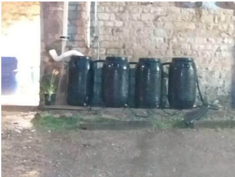
The heavy rainfall in August challenged our temporary downspout solution.
