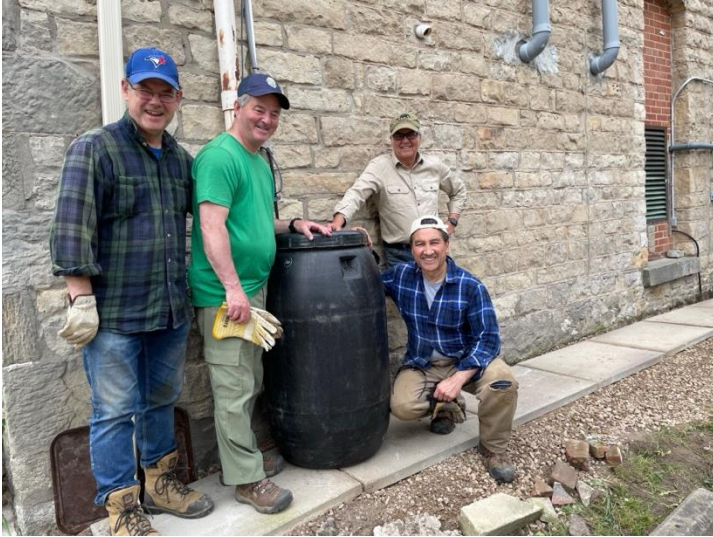
The "crew" after building the base. Bob Abuja, Steve Crocker, Bruce Gregersen, Joe Mauti
