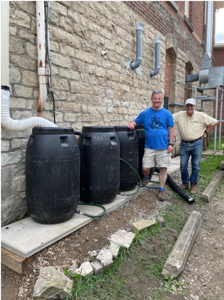
The initial installation of 4 rain barrels by Steve Crocker and Bruce Gregersen
